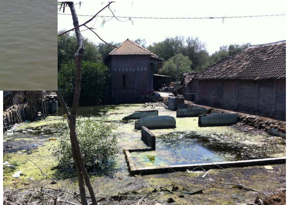
Due to sea level rise and infiltration, some houses in Timbulsloko village are abandoned and moved out
